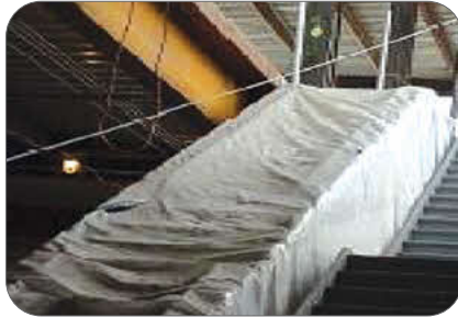
Figure 37: Wire rope lifeline used for fall protection.
