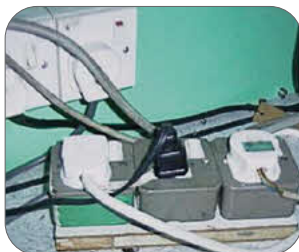
Figure 7: Overloaded circuits and plugs.
