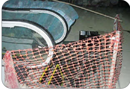
Figure 10: Fall into escalator opening during installation.
