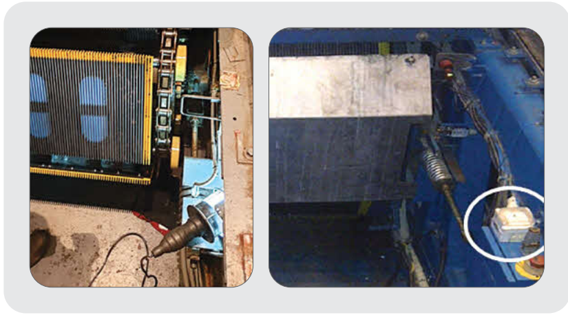
Figure 31: Provision of additional socket for portable light.
