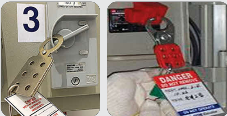
Figure 27: LOTO for the main-line switch of Esc/MW.
