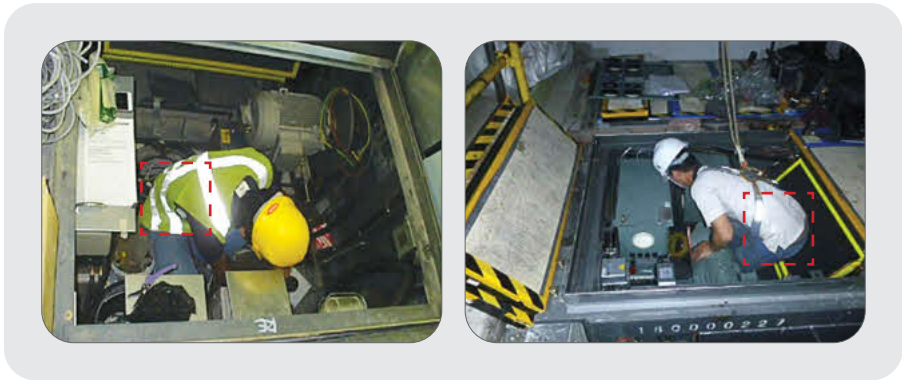
Figure 23: Bad posture due to space constraints.
