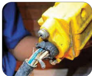
Figure 6: Damaged electrical cords.
