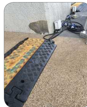
Figure 7: Cable trench covering electrical cables.
