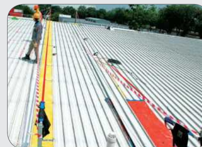
Example of horizontal lifelines on roof.
