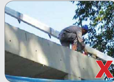
Working on roof without any edge barricade.
