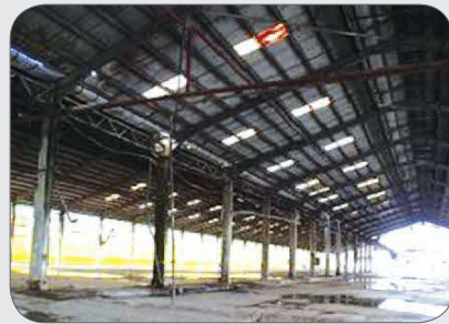
Old Industrial building with skylight and asbestos roof sheets.
