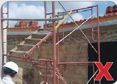
Unsafe scaffold used to access roof.
