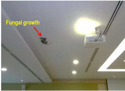
Figure 4: Fungal growth on ceiling board.
