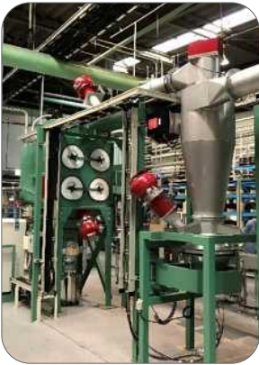
Figure 9: Example of an indoor dust collector with explosion suppression system
