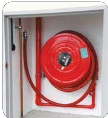
Figure 16: Fire hose reel located inside a cabinet
