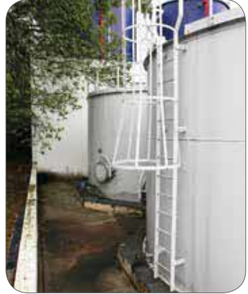
Figure 14: Example of a diked storage area
