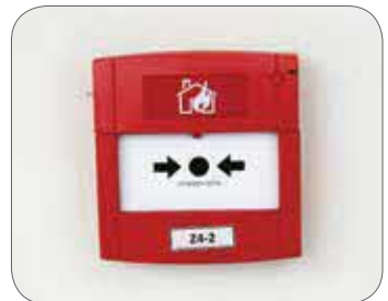
Figure 13: Fire Alarm Call Point
