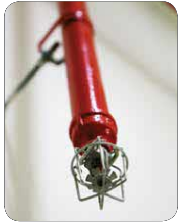
Figure 17: Standard sprinkler with guard
