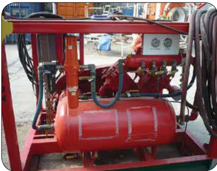
Figure 17: Typical LP air compressor.
