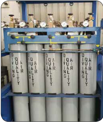
Figure 9: HP cylinders in quads.
