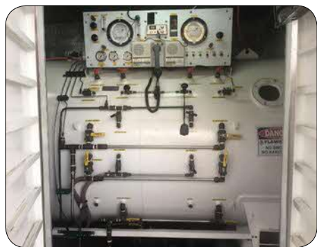
Figure 15: DDC (external) with control panel.
