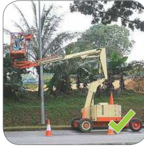
Figure 47: MEWP must be stably positioned to avoid hazards such as toppling.
