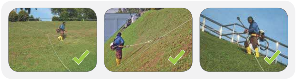
Figure 28: Install proper anchorage to railings using Self-Retracting Lifeline (SRL) or other protection method is to prevent fall.
