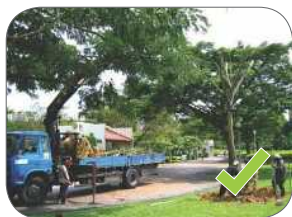
Figure 49: Workers face the risk of being hit by falling or swinging loads during crane operations.
