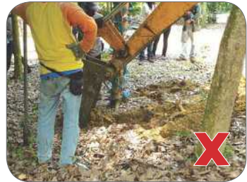
Figure 54: When the excavator is in operation, no one shall enter the full swing area of the machine.
