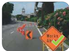
Figure 51: Place warning signs to re-direct other road users.
