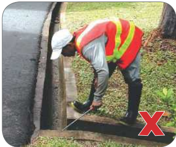
Figure 105: When a worker needs to bend down to clear the drains.
