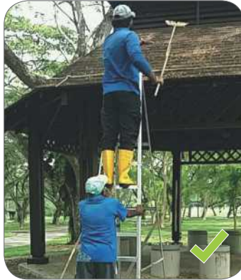
Figure 4: Place ladder on level and firm ground, and get another worker to hold it firmly. Refer to Section 2.3.1 under Part A on safe use of ladder.
