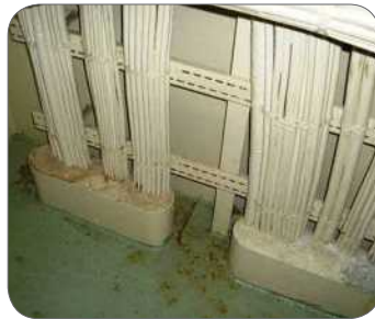
Figure 4: Asbestos-containing cable penetrations used on ships.
