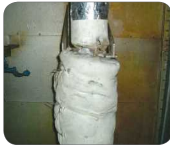
Figure 3: Asbestos cloth wrapping with asbestos lagging of exhaust pipe.
