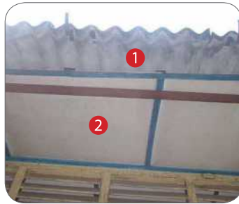
Figure 2: Asbestos used in building roof sheets and ceiling boards.
