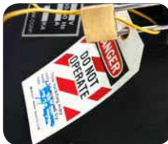
Figure 8: Machine locked-out and tagged-out for maintenance.
