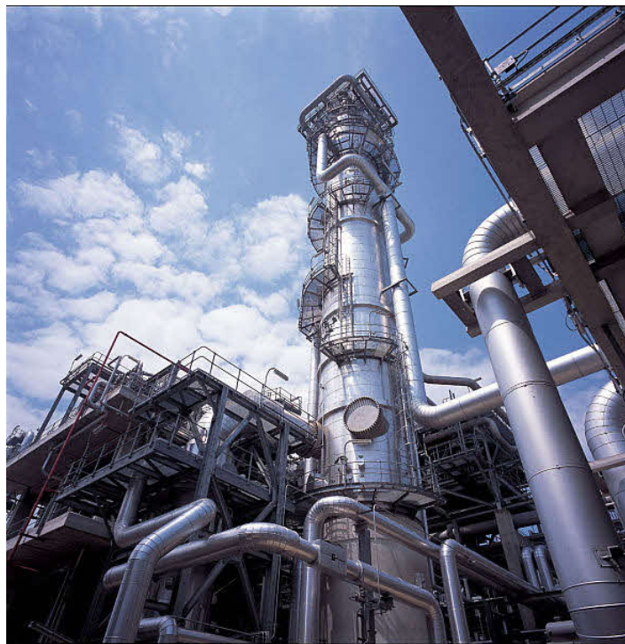
Figure 4: A typical column in a chemical plant
