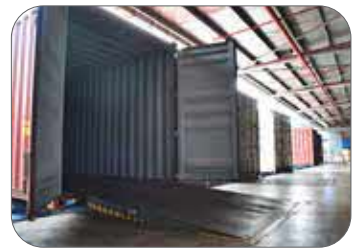
Figure 7: Dock leveller (integrated to loading dock).
