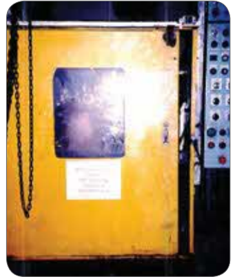
Figure 33: Sliding door was not fitted with an interlocking guard.
