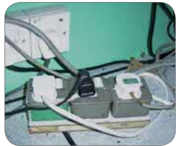
Figure 12: Haphazard electrical connections can lead to overloading and electrocution.
