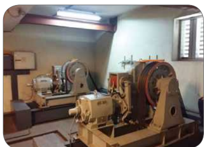
Figure 63: Clean, tidy and bright motor room
