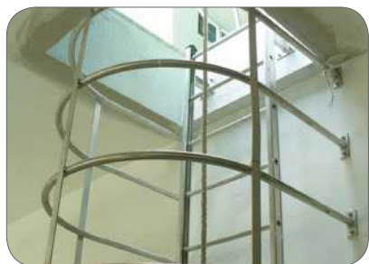
Figure 53: An example of ladder with safety cage
