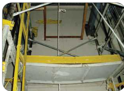
Figure 35: Falling off from improperly constructed platform
