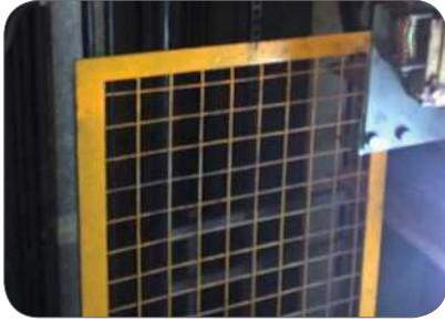
Figure 39: Multiple hoist ways and car top
