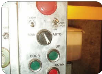
Figure 81: Operational switch set to maintenance
