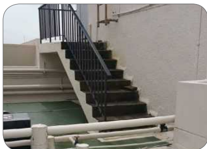
Figure 43: Motor room access with obstruction
