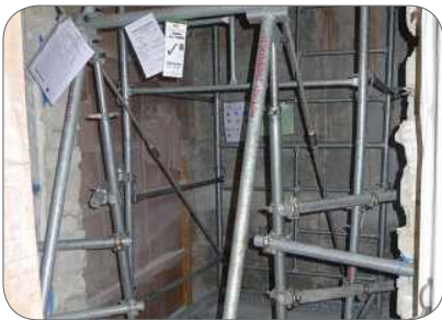
Figure 30: Falling off from cantilevered scaffold
