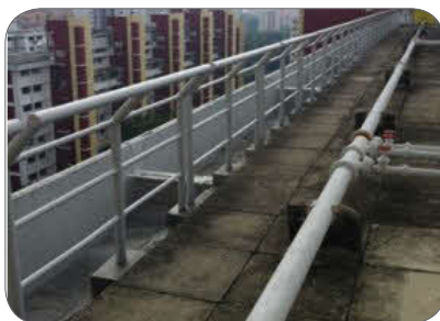
Figure 59: An example of roof top safety railing
