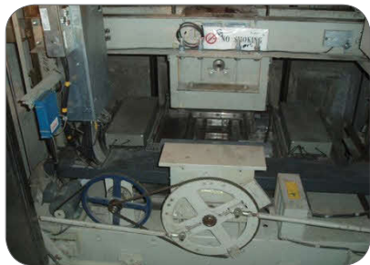
Figure 80: Car positioned near landing
