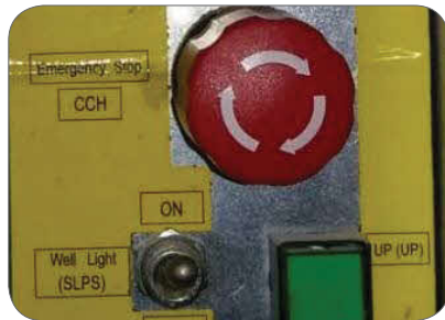
Figure 70: Emergency stop switch at lift motor room
