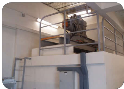
Figure 67: Safety railing to prevent falling from height
