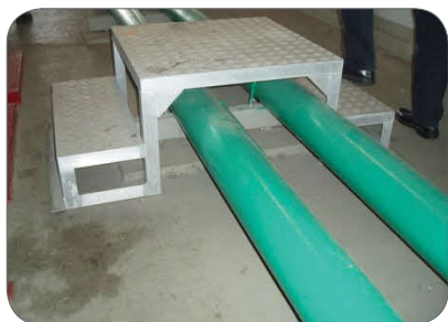
Figure 58: An example of access platform over pipes
