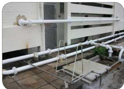
Figure 42: Motor room access with obstruction
