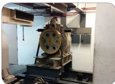
Figure 64: Motor room with ventilation system
