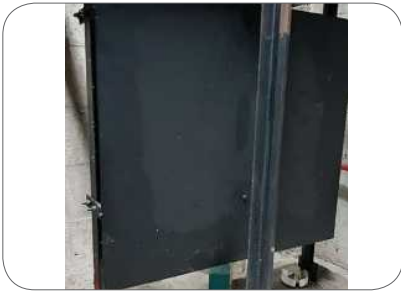
Figure 89: Counterweight screen installed in lift pit
