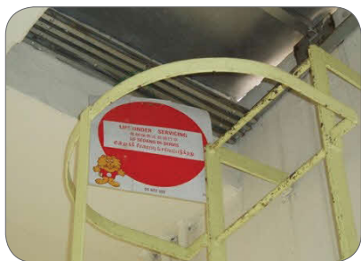
Figure 57: Display notice of lift maintenance in progress
