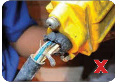
Figure 20: Damaged electrical cords
