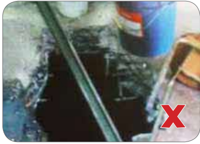
Figure 29: Potential fall hazard—floor openings in motor room.
