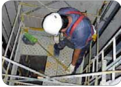
Figure 28: Falling off metal scaffolds.
