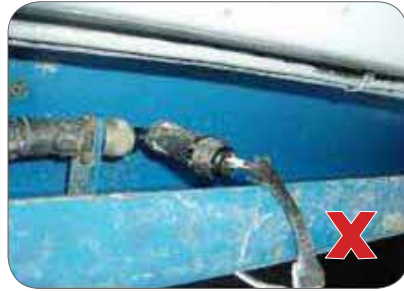
Figure 11: Damaged electrical cords.
