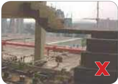
Figure 21: Falling off the unprotected edge of stairs.
