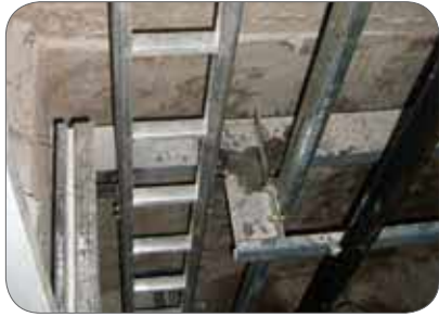
Figure 31: Falling off pit ladders.
